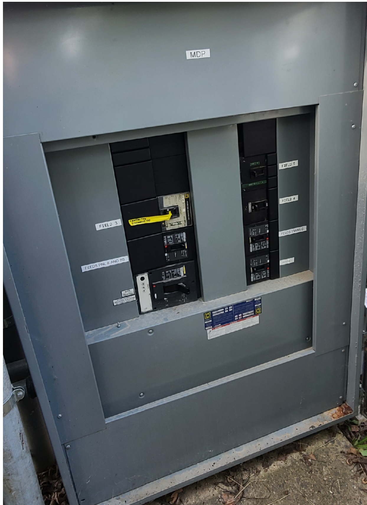
5 EXISTING MAIN DISTRIBUTION PANEL LOCATED BEHIND FIELD 3 E1.0 NO SCALE
