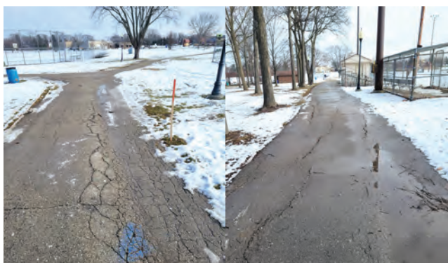
PATHS WITH ASPHALT ISSUES, RUTTING & CRACKING.
