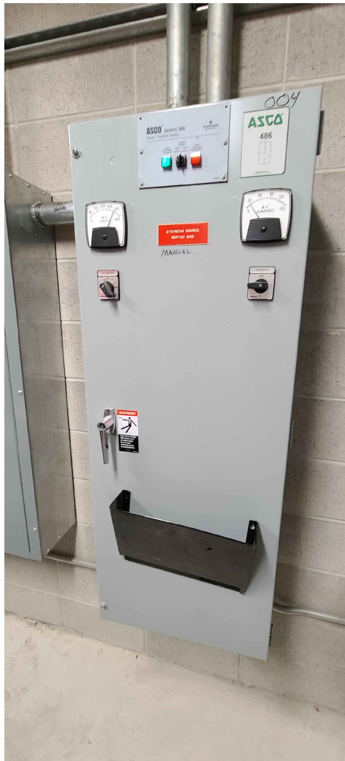
4 EXISTING MANUAL TRANSFER SWITCH "NEHA" SCALE: NTS
